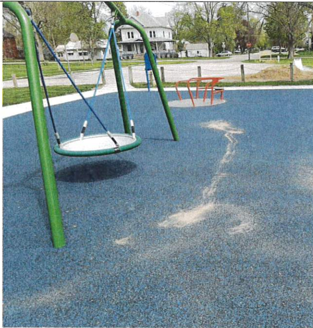
Project 3, Tactic 2: One of the challenges we've experienced is needing to clean the surface after things like these piles of sand were dumped.
